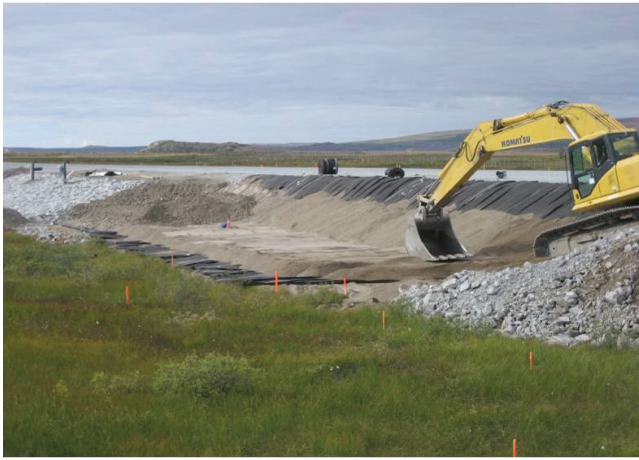
Figure 1. Installation of the heat drain in the shoulder of the Tasiujaq airstrip embankment.
